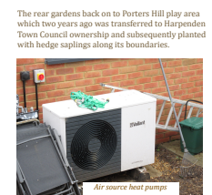
Air source heat pumps
